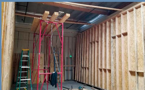
The interior frame is in place as the room begins to take shape.
